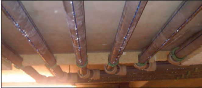
Illustration 6.5 Condensation on cold water lines
